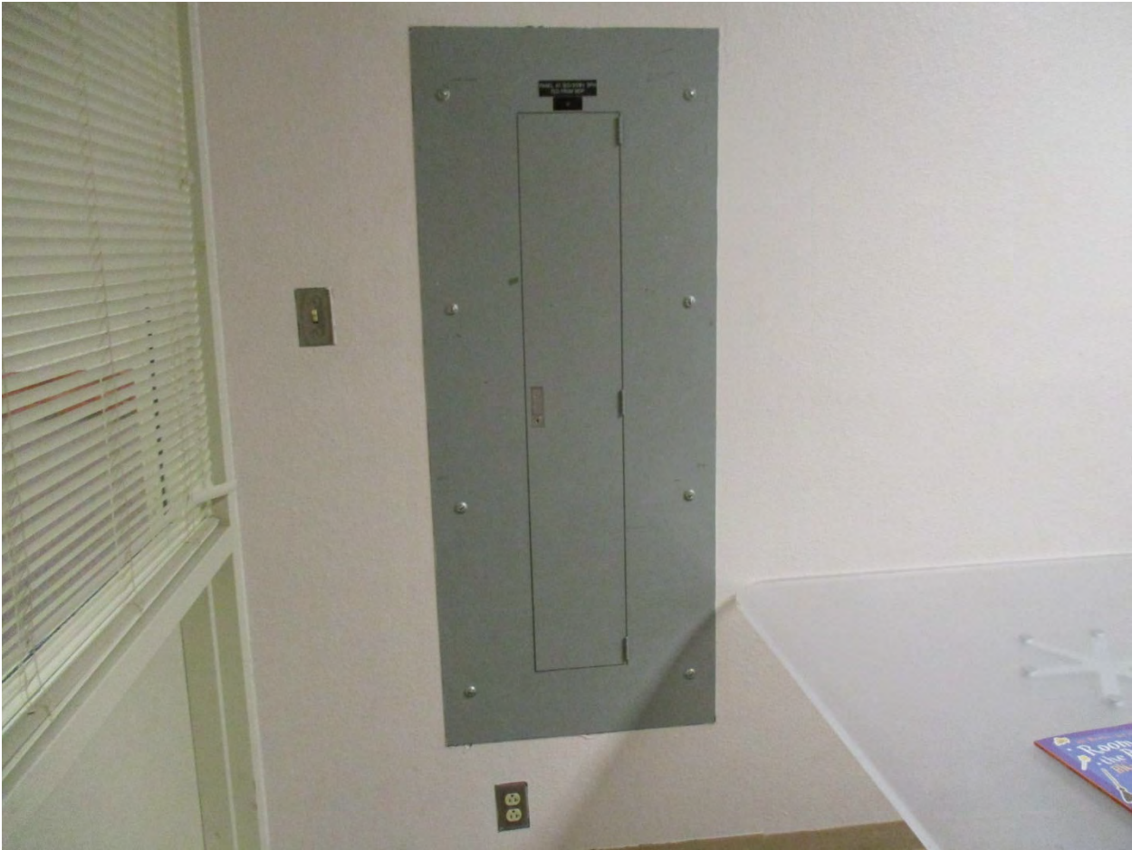
Accessible electrical panel in elementary school hallway
